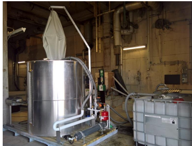
Biogas unit, operated by Tampere University of Technology
